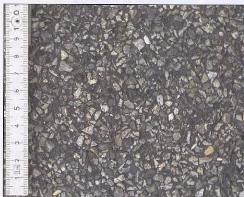
Fig. 21.12 Epoxy-durap surface dressing on a cement concrete surface. Road A270 near Nuenen, the Netherlands.
